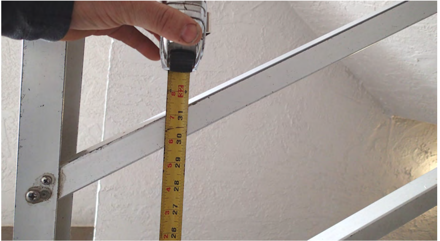
Figure 3: Typical stair grab rails too low. Height should not be less than 34”.
