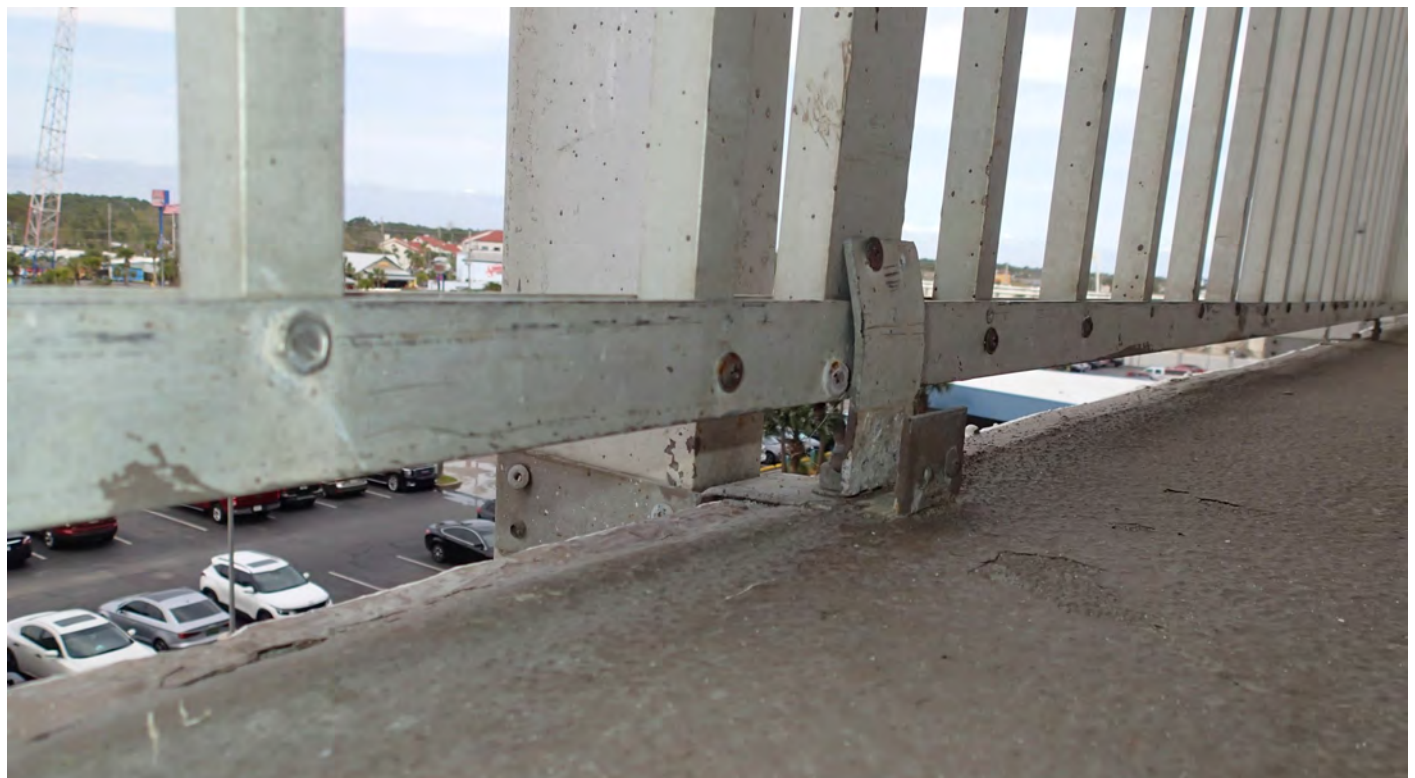
Figure 6: Typical handrail connections are modular, and rely on screws and rivets for connections. Many fasteners are broken, loose, and missing.
