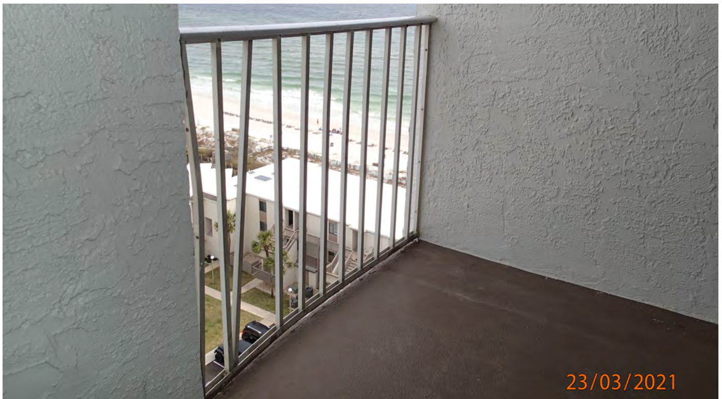
Figure 8: Damaged end rail with broken picket.
