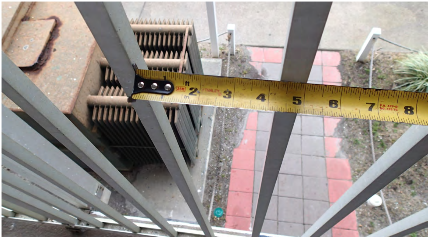
Figure 2: Typical picket spacing on all handrails in excess of code maximum 4".
