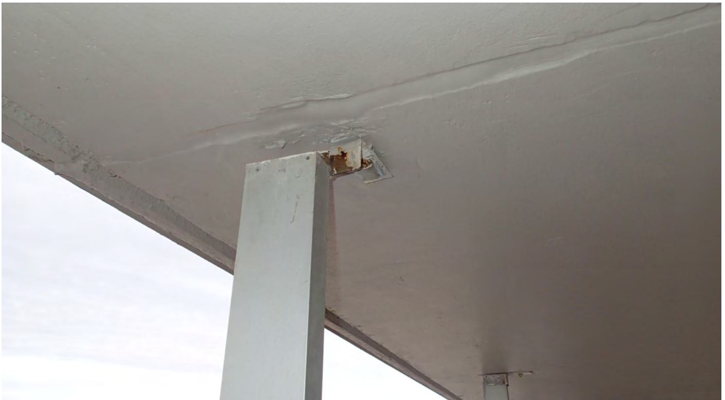
Figure 10: 15th floor—Connections at the top of main support columns. Some are loose or broken.
