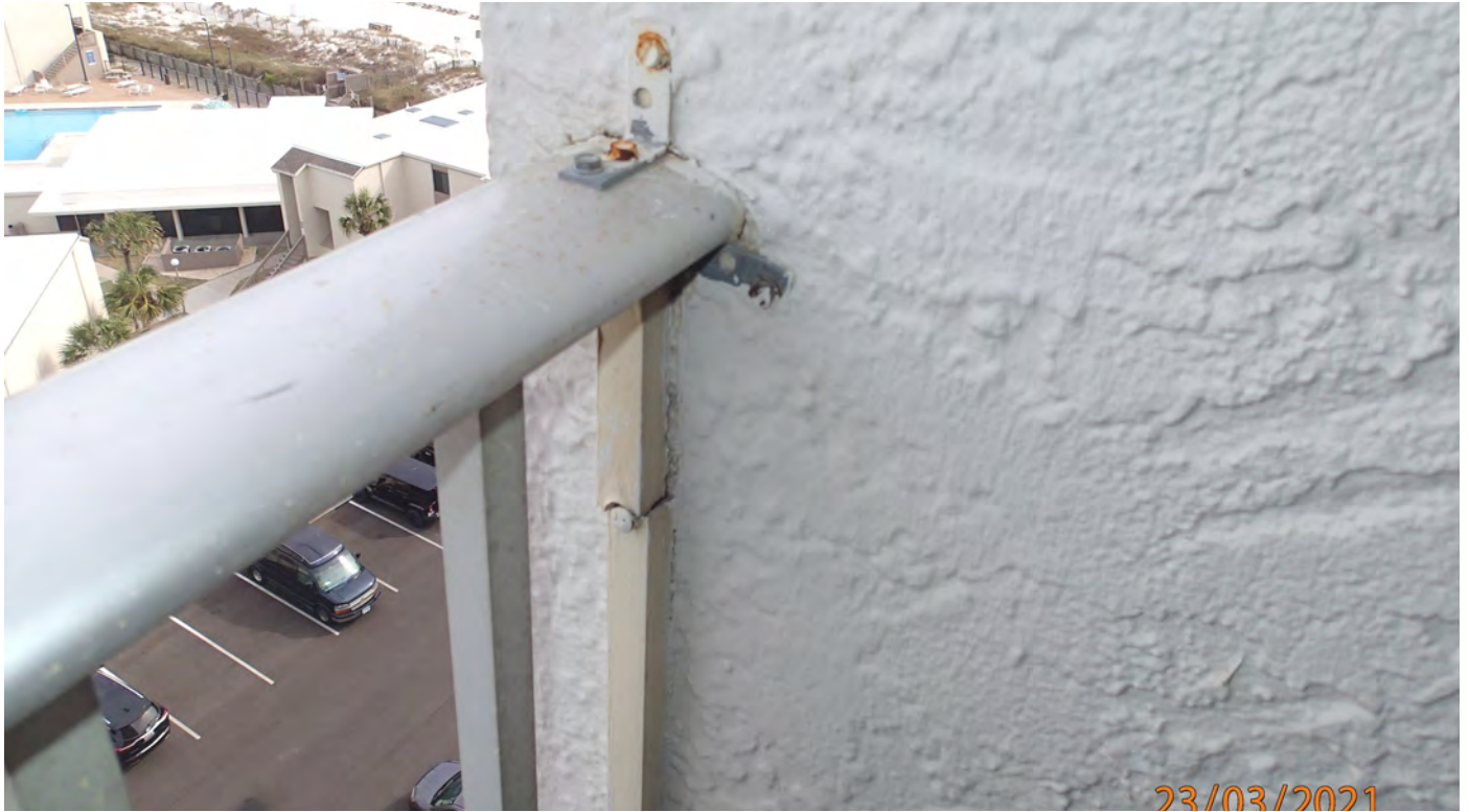
Figure 9: Typical repairs on handrails are insufficient.
