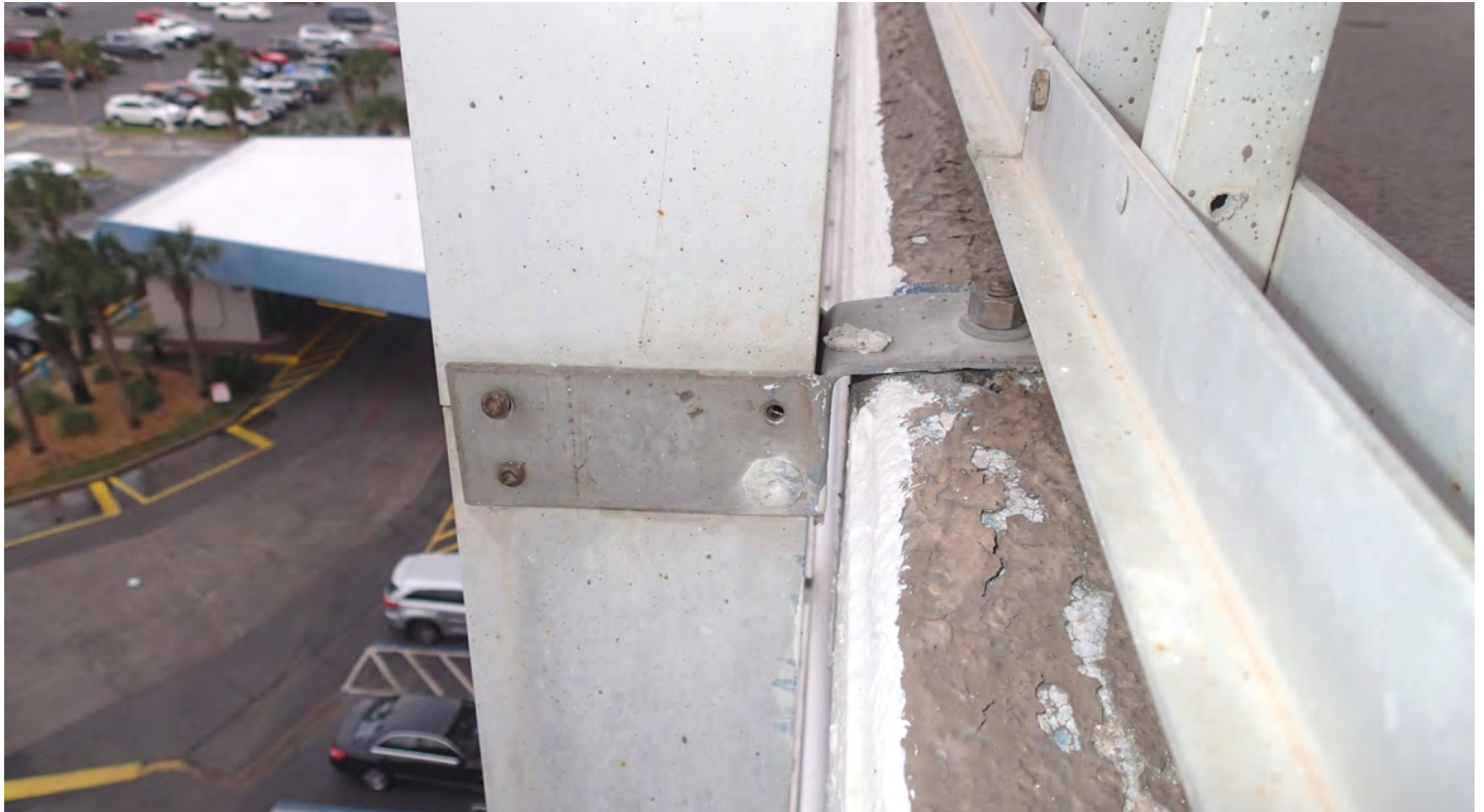
Figure 7: Typical main column connections to building with missing and broken screws.
