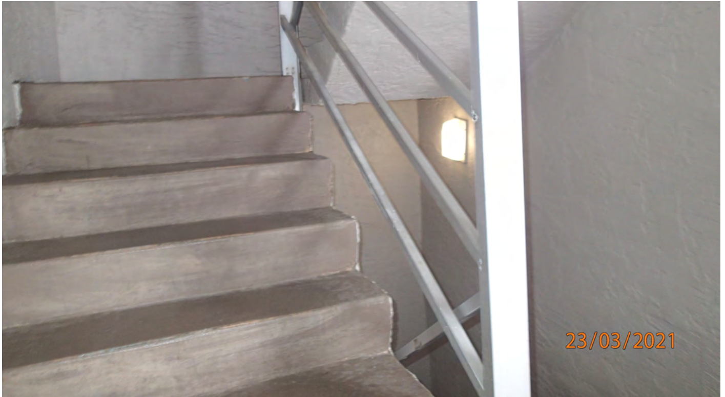
Figure 11: Most stairs do not have ant-slip surface on treads. Inspection was done during a rain event. Stairs are slippery when wet.
