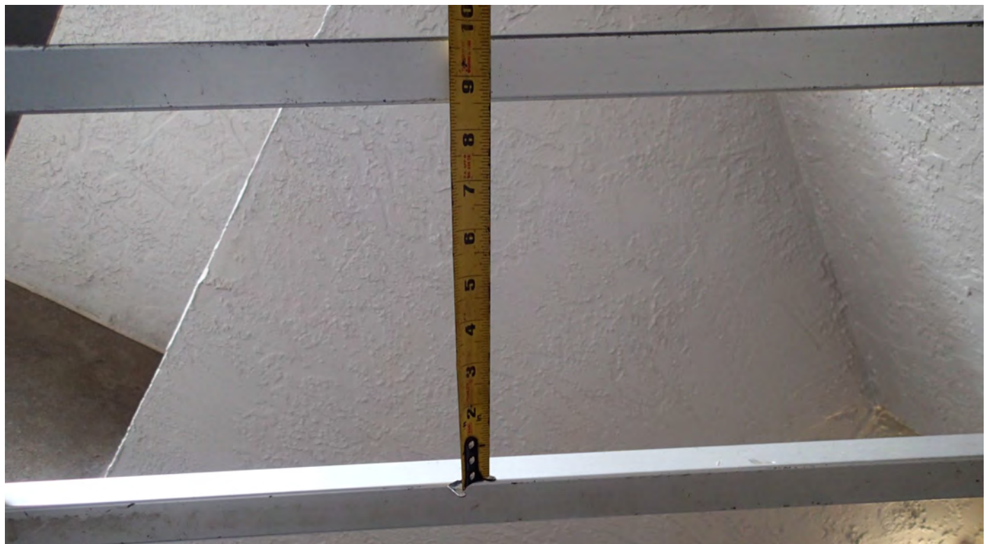
Figure 4: Handrail spacing too large on stairs. Maximum 4”, 6” at triangle at stair tread.
